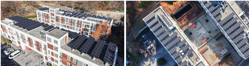
Rooftop solar power installation at Yanghak Town in Pohang
